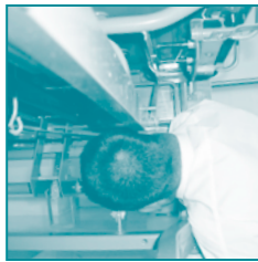
Bed frames should be checked to assure safety stops are in place to minimize crush risk to patients.
