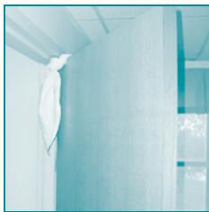
A knotted sheet can serve as a hanging risk when combined with solid core hospital doors on inpatient psychiatric units.
